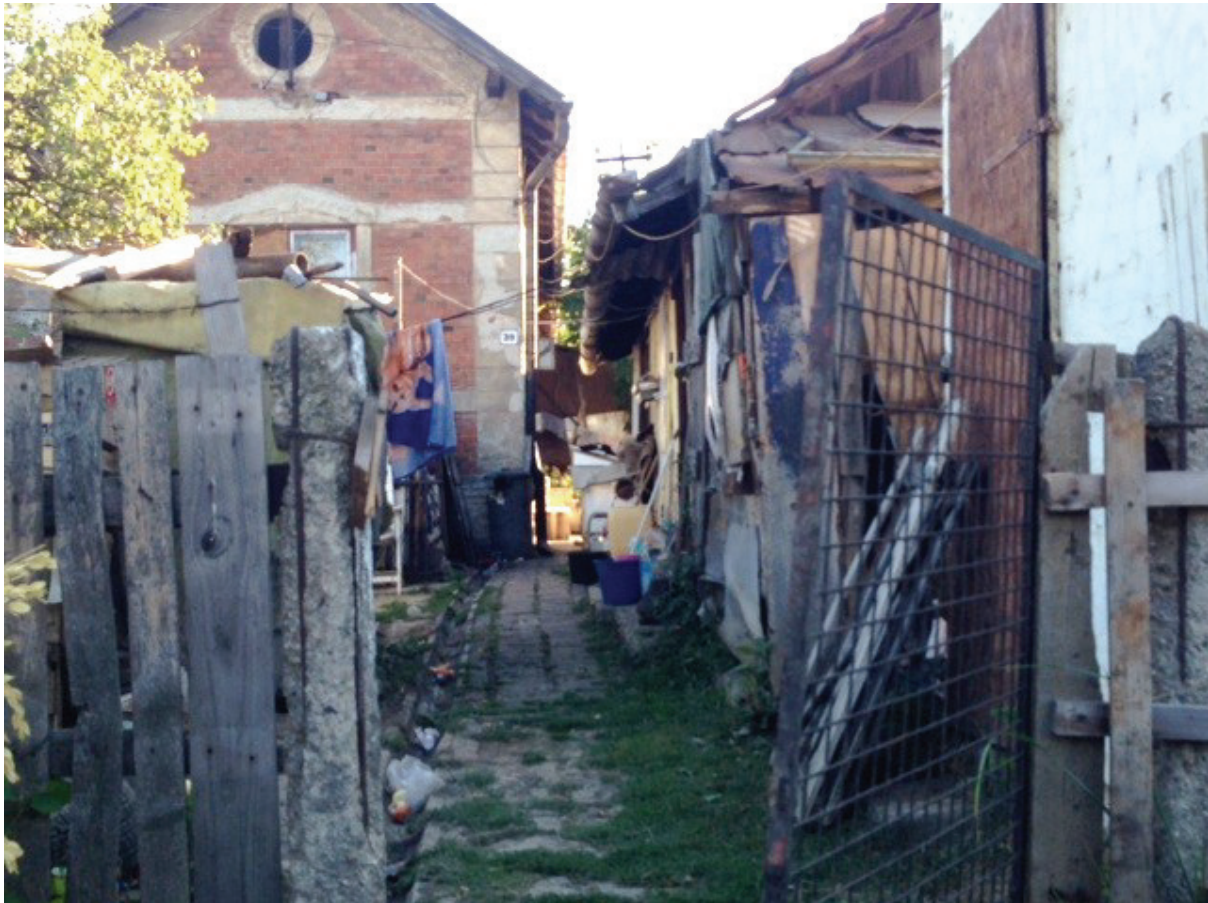
Figure 1. Architectural, public health and epidemiological state of the dwellings were unacceptable. Buildings leaked, the walls were damp and mouldy. Hygienic facilities (running water; bathroom), proper ventilation and modern heating possibilities were all lacking.
